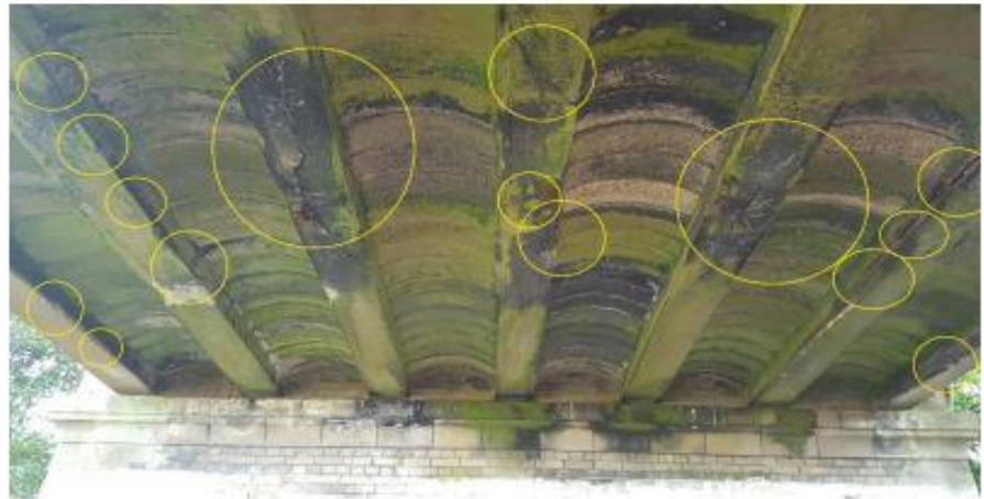
Concrete encasement around each beam had also fractured (highlighted) and spalled.
