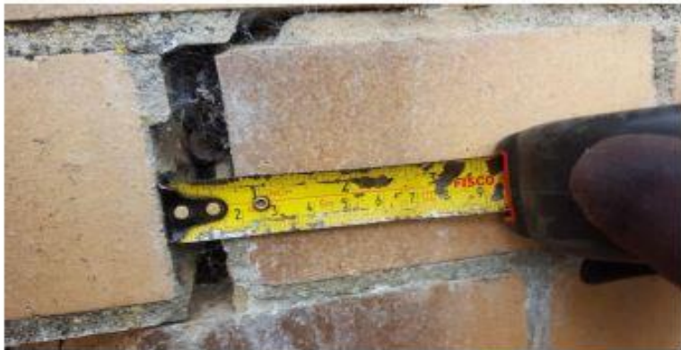
Close up photo of fracture in north side abutment, fracture measuring 25mm.
